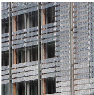
Semi-transparent modules integrated into louvres - Le Albere, Trento (Italy) Photo: S. Croce
