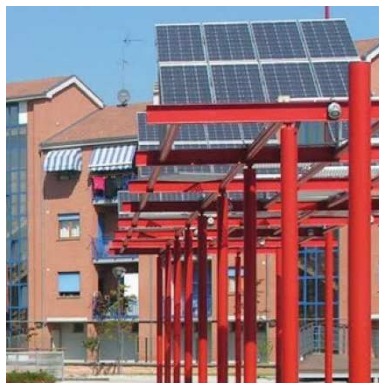
PV pergola - Violino photovoltaic village, Alessandria (Italy)
